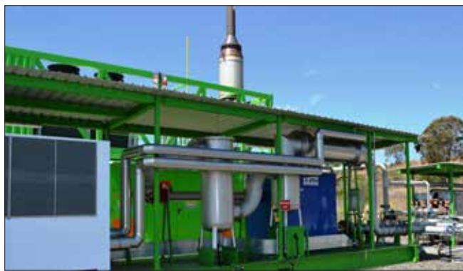
LEFT: Gas cleaner skid that cleans the methane that comes from the Hermitage Road landfill 2km away, before entering the generator
